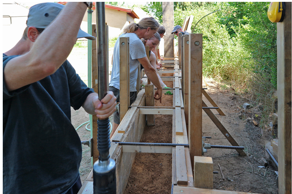
15 Rammed earth workshop, European Training Centre for Earth Building in Wangelin, D
