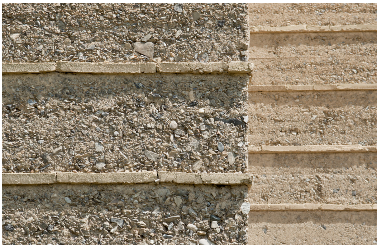
12 Calculated erosion: The weather-exposed facade of the Rauch House after two years of erosion
