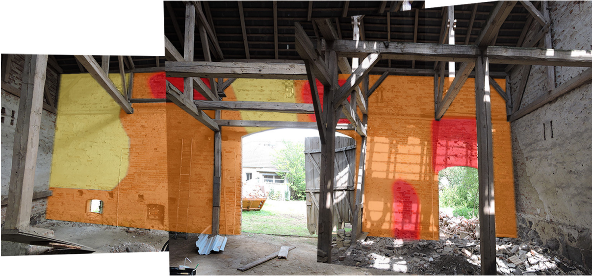
07b Barn in Weesow, D: Interior with areas of supercritical salt contamination marked
