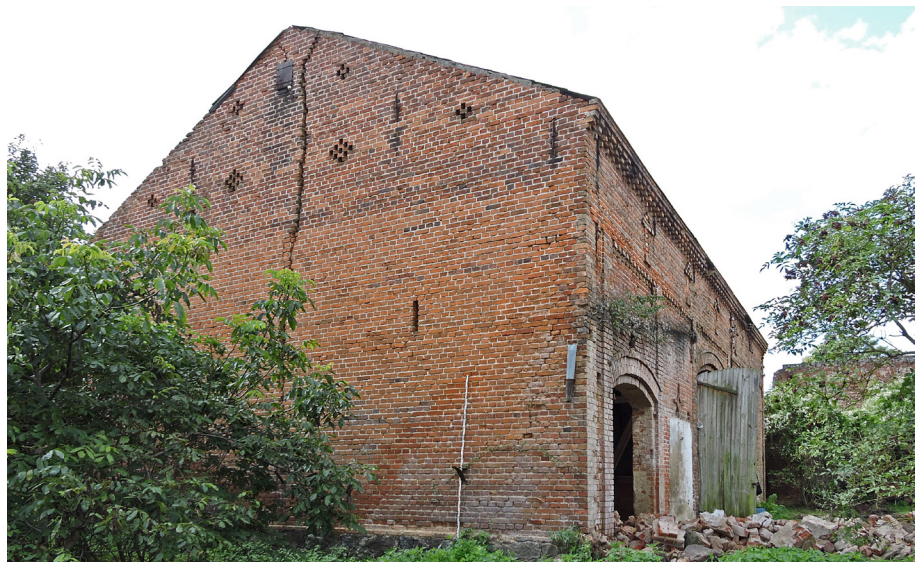
07a Barn in Weesow: View from outside showing clearly visible moisture and salt damage.
