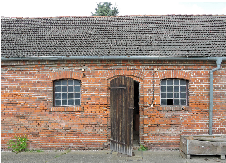
01 Former stable building with clear indications of moisture and salt load on the brickwork
