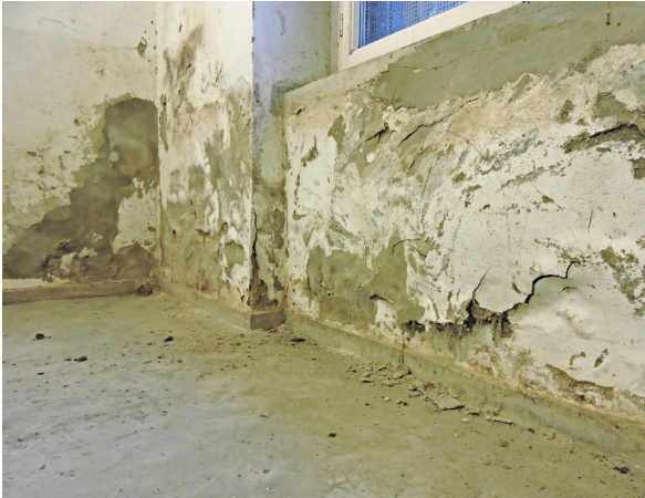
02 Restoration plaster after a service life of 10 years without installation of a horizontal barrier
