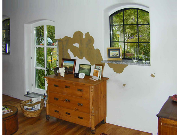
04 Even after installing a horizontal damp proof course, damage can still occur if no salt reduction measures are undertaken
