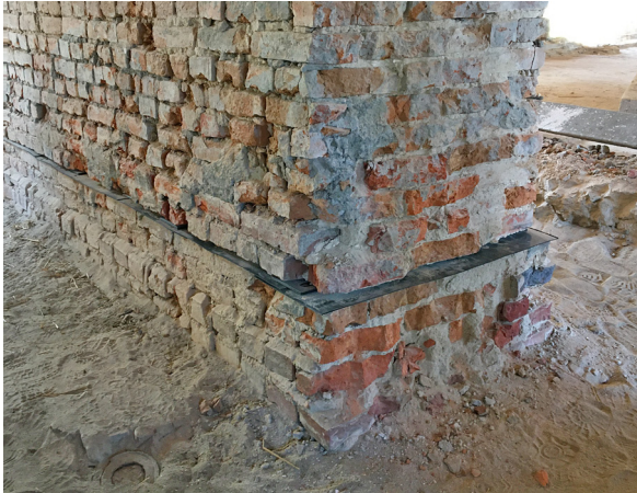
05 Installation of a mechanical horizontal barrier using the wall sawing method as a preparatory measure for desalination
