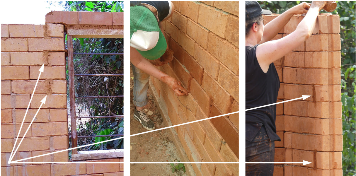
08 To stop the liquid grouting escaping through the vertical joints between blocks, especially when halved manually on site, the gaps must be closed with a thick laterite mortar (see arrows)
